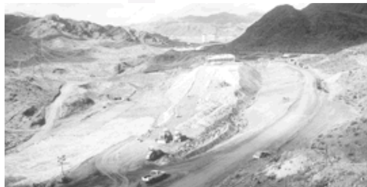
Site work progresses on the Nevada Interchange which includes ramps and a 160-foot-long bridge.
