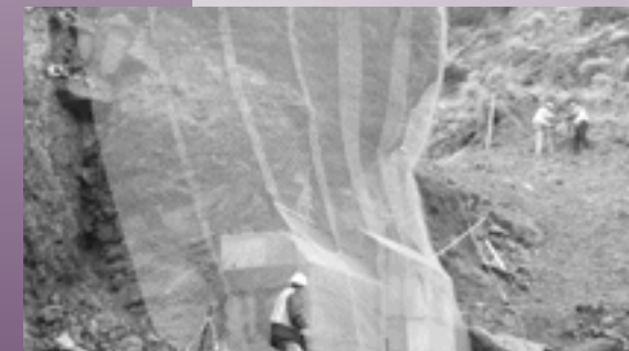
Crews wrap containment fencing around rock prior to blasting near the Colorado River Bridge abutment.
